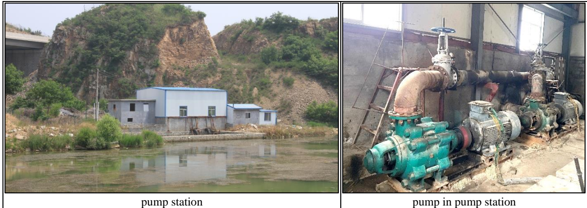
Figure 16-5: Pump Station for Processing Production
