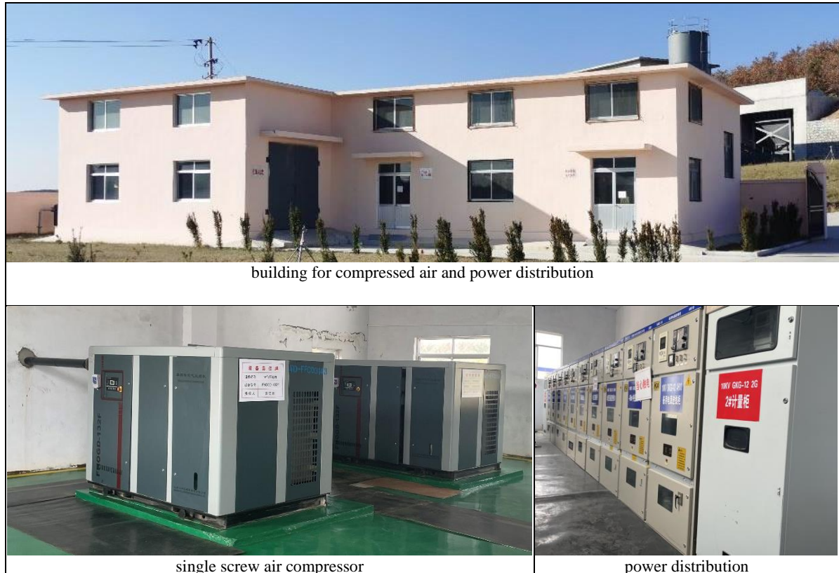
Figure 14-8: Compressed Air Station and Power Distribution Room
