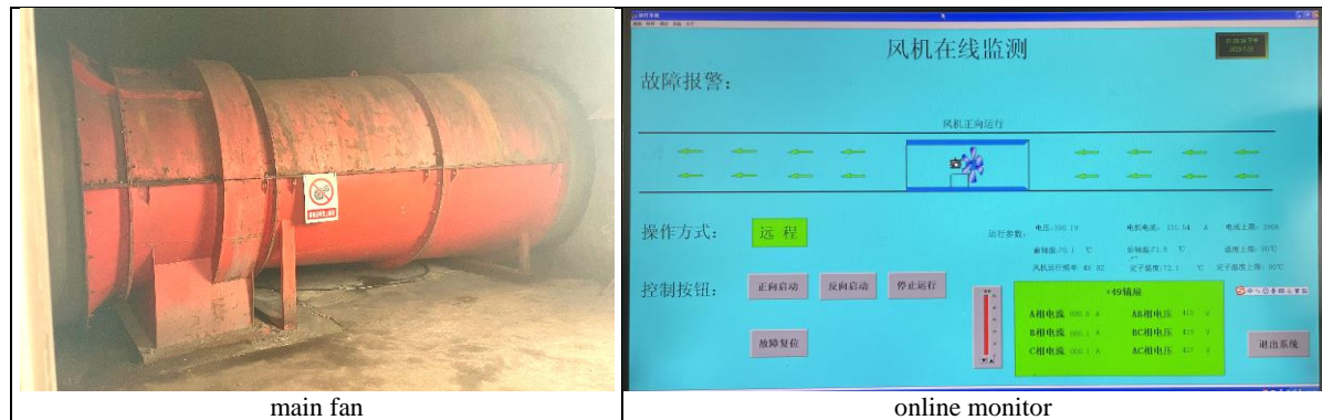
Figure 14-6: Main Fan at the Portal of Upcast
