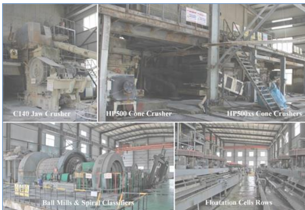
Figure 15-6: Photos of Processing Equipment
