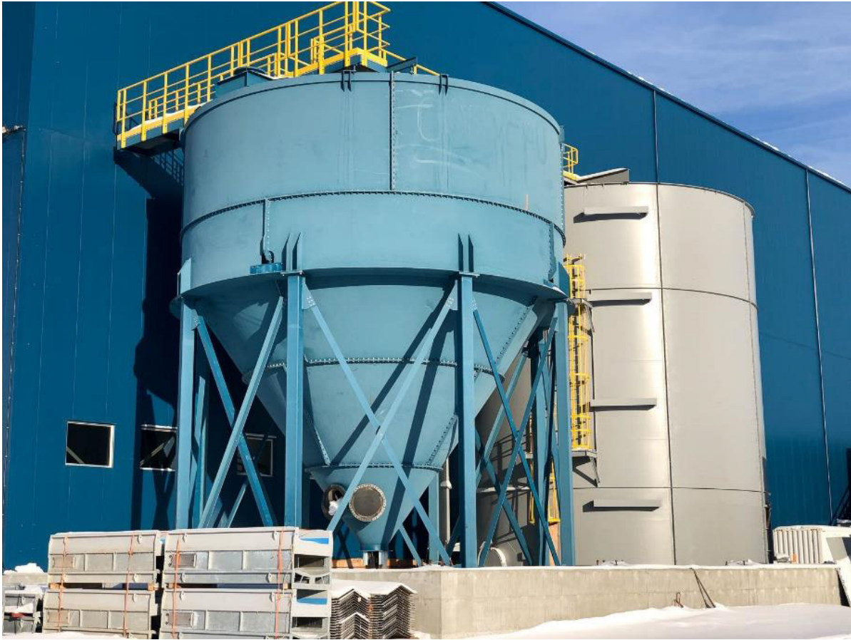
Figure 24-7 View of the Process Water Tank and Thickener Area
