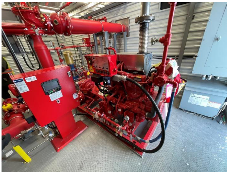
Figure 18-4 Fire Water Pumping Module
