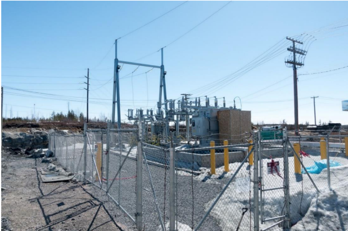
Figure 18-11 Existing Transformer Bay at Whabouchi Mine (69/4.16kV)
