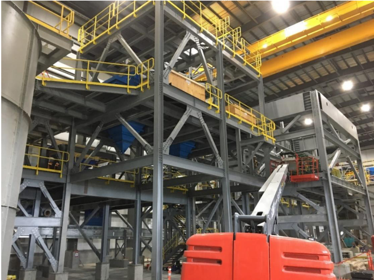
Figure 24-10 View of the Hydraulic Separators
