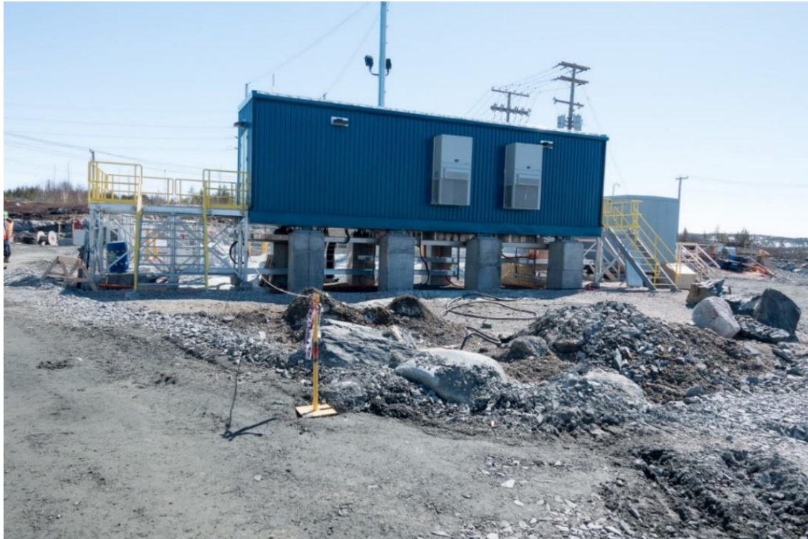
Figure 18-13 4.16 kV Switchgear Building
