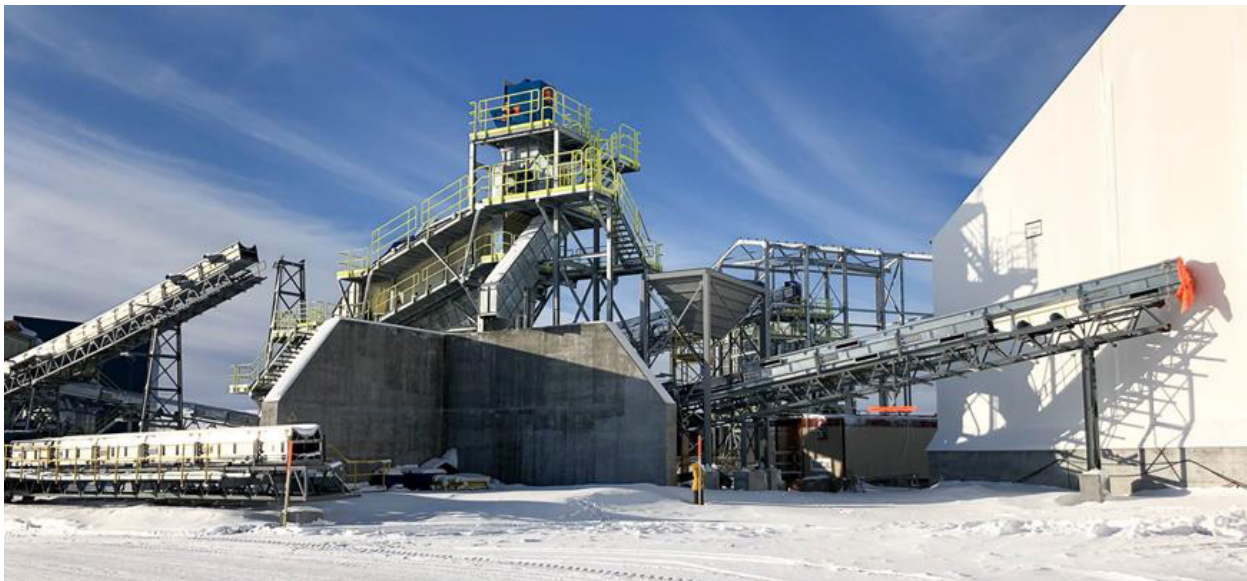
Figure 24-2 View of Screening Tower and Concentrator
