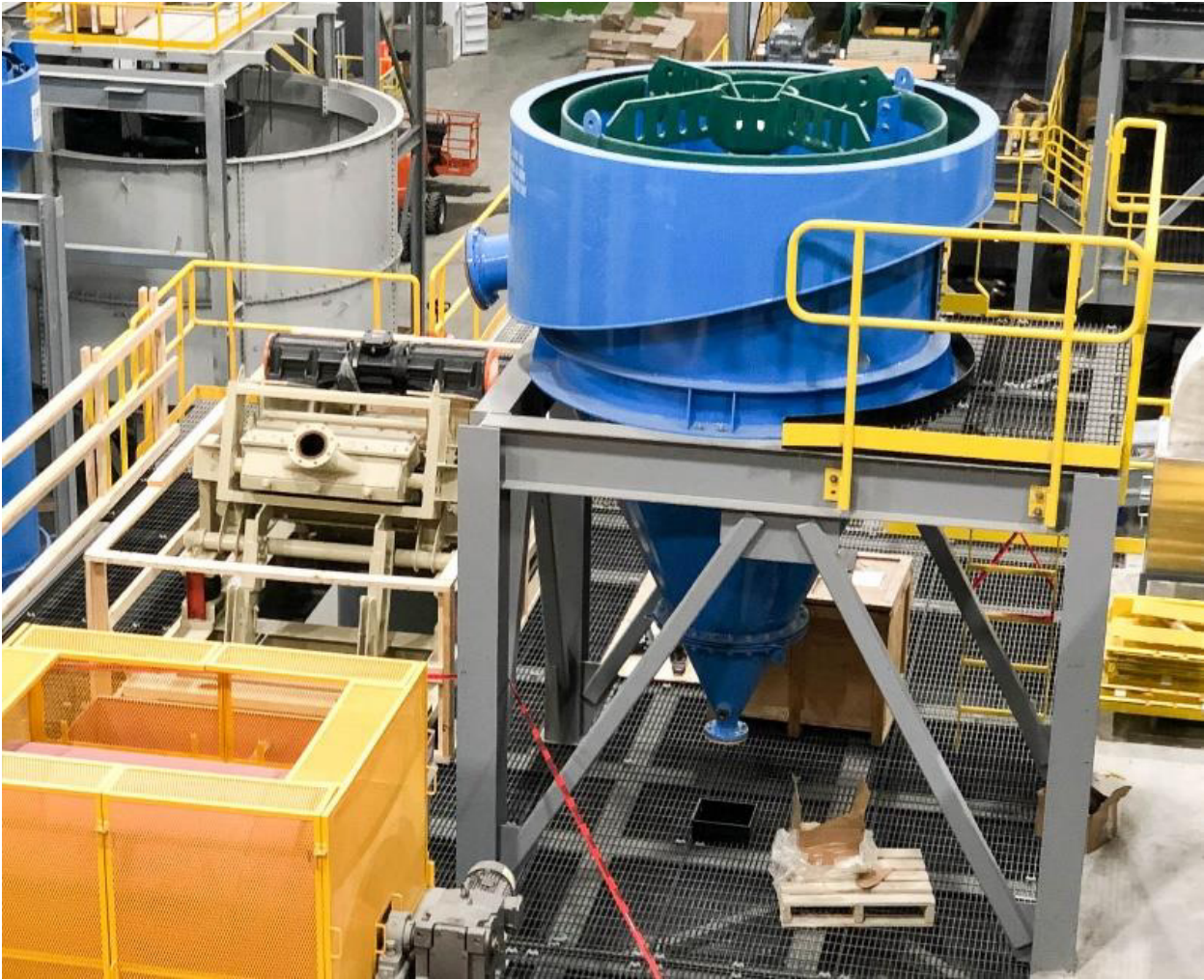
Figure 24-9 View of the Hydrocyclone
