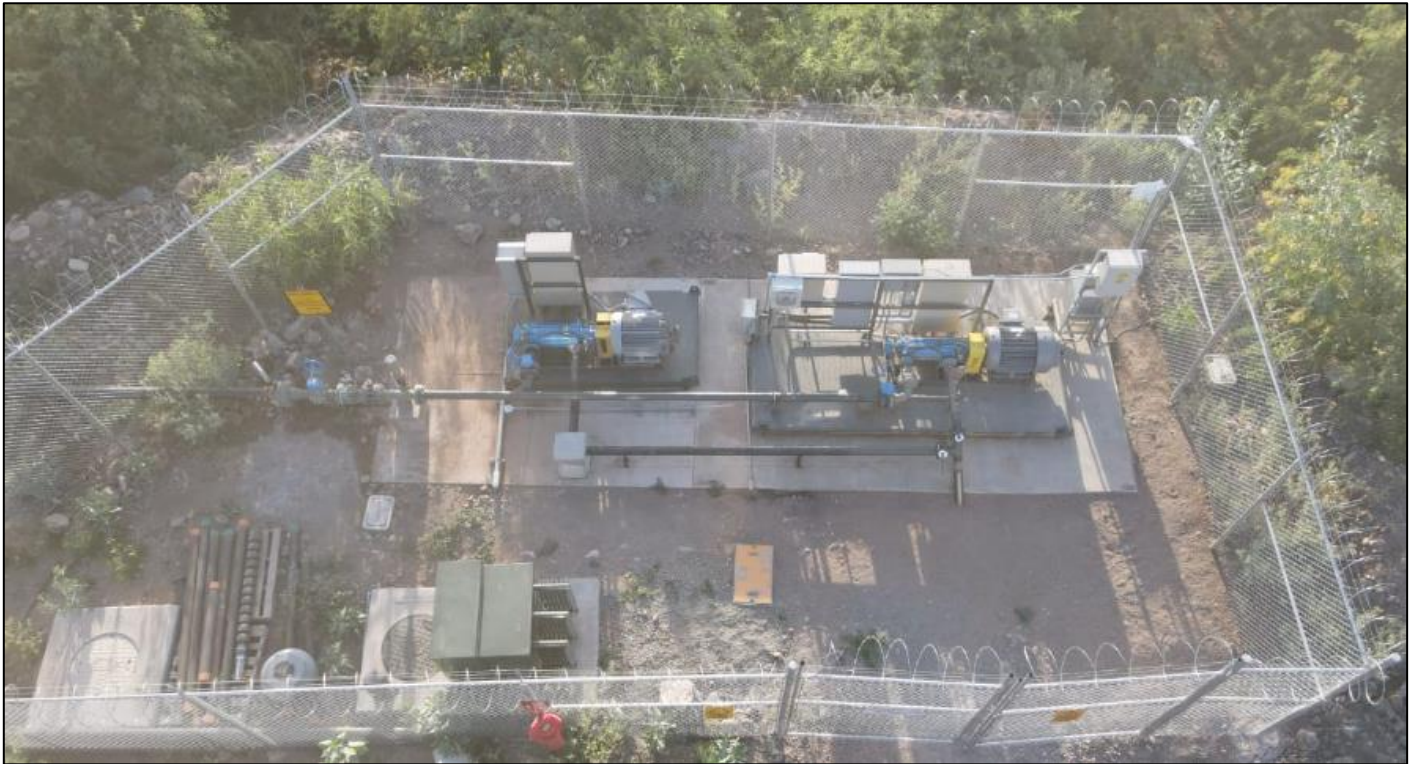
Figure 5-3: Sonora River Pumping Station
