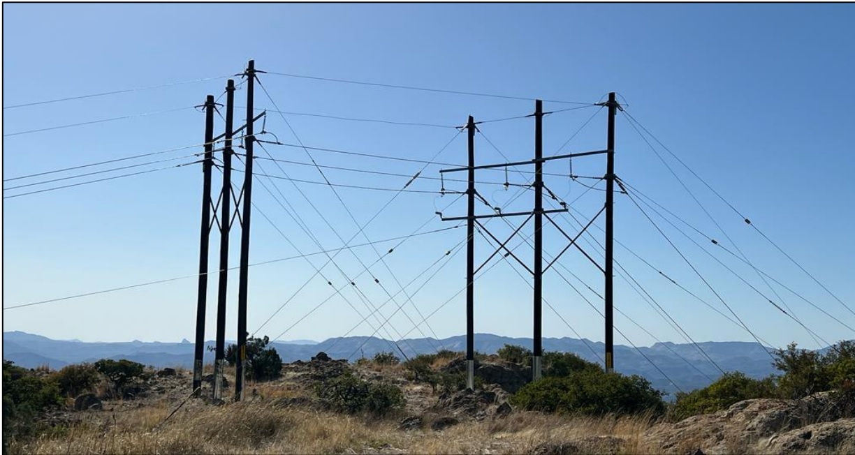
Figure 18-9: Electrical Power Line
