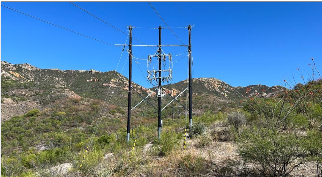
Figure 18-10: Electrical Power Line
