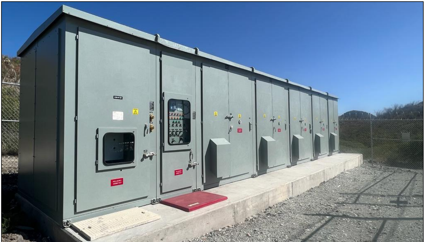
Figure 18-11: Power Equipment for 33 kV Line
