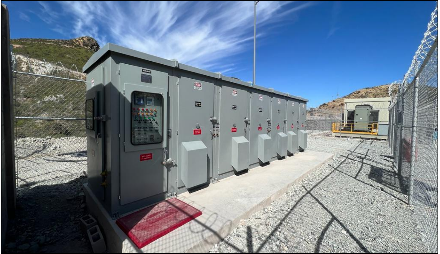
Figure 18-12: Power Equipment for 4.16 kV Distribution Bus
