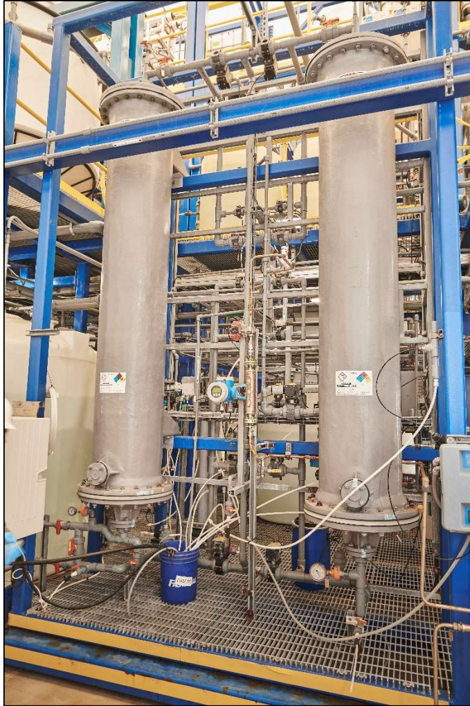
Figure 13-9. Calcium and Magnesium Ion Exchange System at the Demonstration Plant
