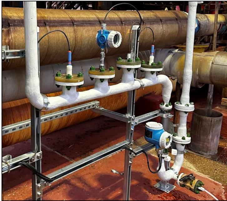
Figure 13-3. Tail Brine Measurement Skid at the LANXESS Bromine Tower
