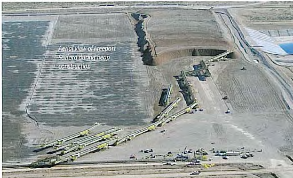
Figure 14-9: Grasshopper conveyors and stacker
