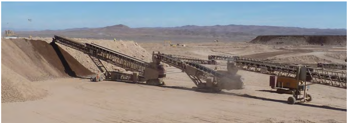
Figure 14-8: Grasshopper conveyors and stacker
